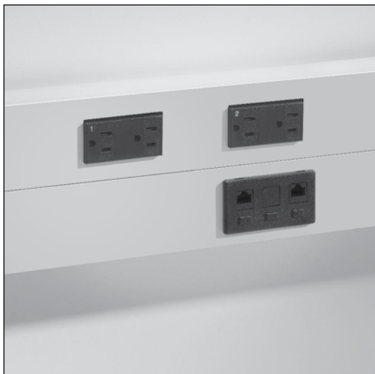
Standard Vox Power Channel configuration 2-duplex receptacles, 1 Data, 1 Blank, 1 Voice
